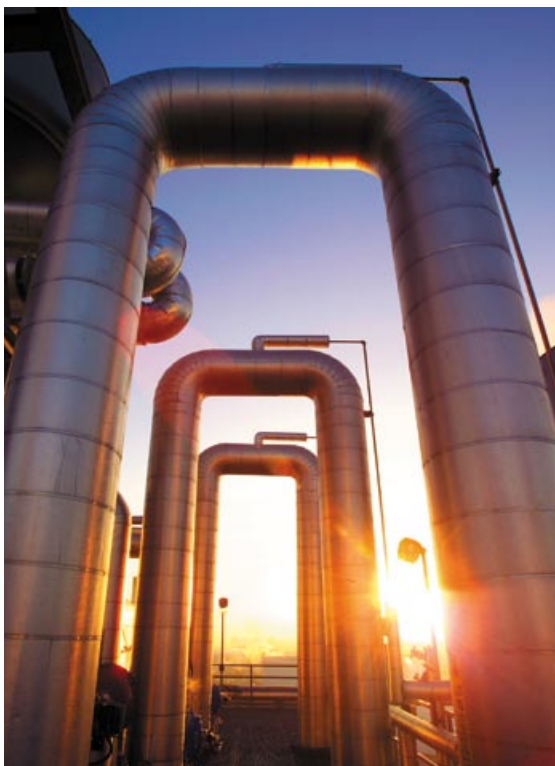
Photo courtesy of Calpine Corporation
